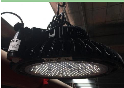
XSY LED high bays with VABOSS smart controls
